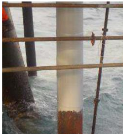
Figure 1.0: Condition of splash zone area after composite wrapping application
