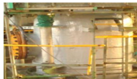
Figure 2.0 shows the condition of the deaerating vessel after application of rehabilitation system
