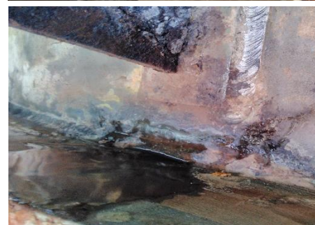
Figure 1.0 shows the defect point of the deaerating vessel
