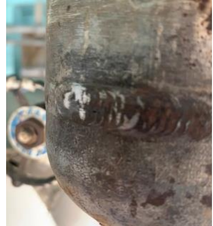
Figure 1.0: Defect on the pipe – crack line leak at weldment
