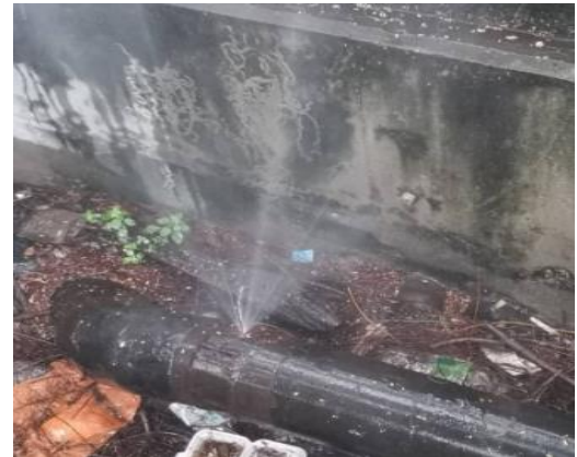
Figure 1.0: Condition of initial defect
