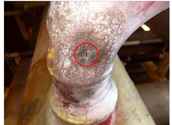
Figure 1.0: Initial condition of 3” elbow pipe
