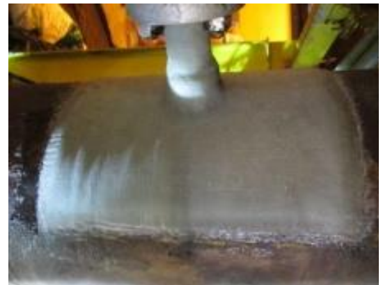
Figure 2.0: Visual of applied repair system on the 1.5” flangeolet prior to topcoat application
