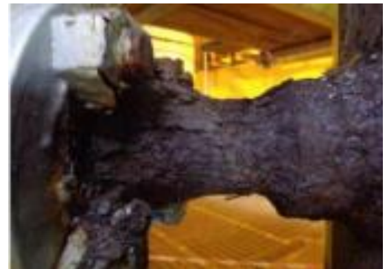
Figure 1.0: Initial condition of 1.5” flangeolet
