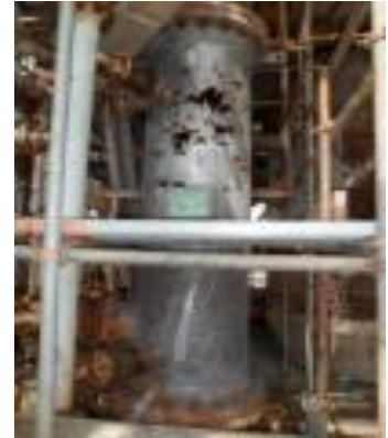
Figure 1.0: Condition of the leak prior to repair application
