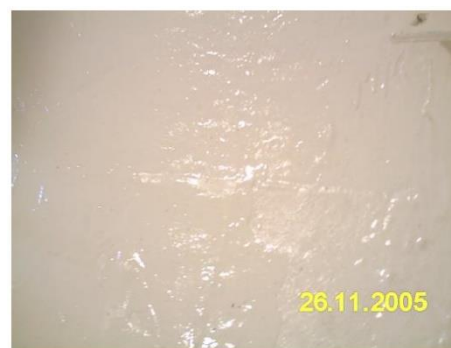
Figure 2: Close-up view of the Corro Dur Wet Lay-Up system applied in the tank
